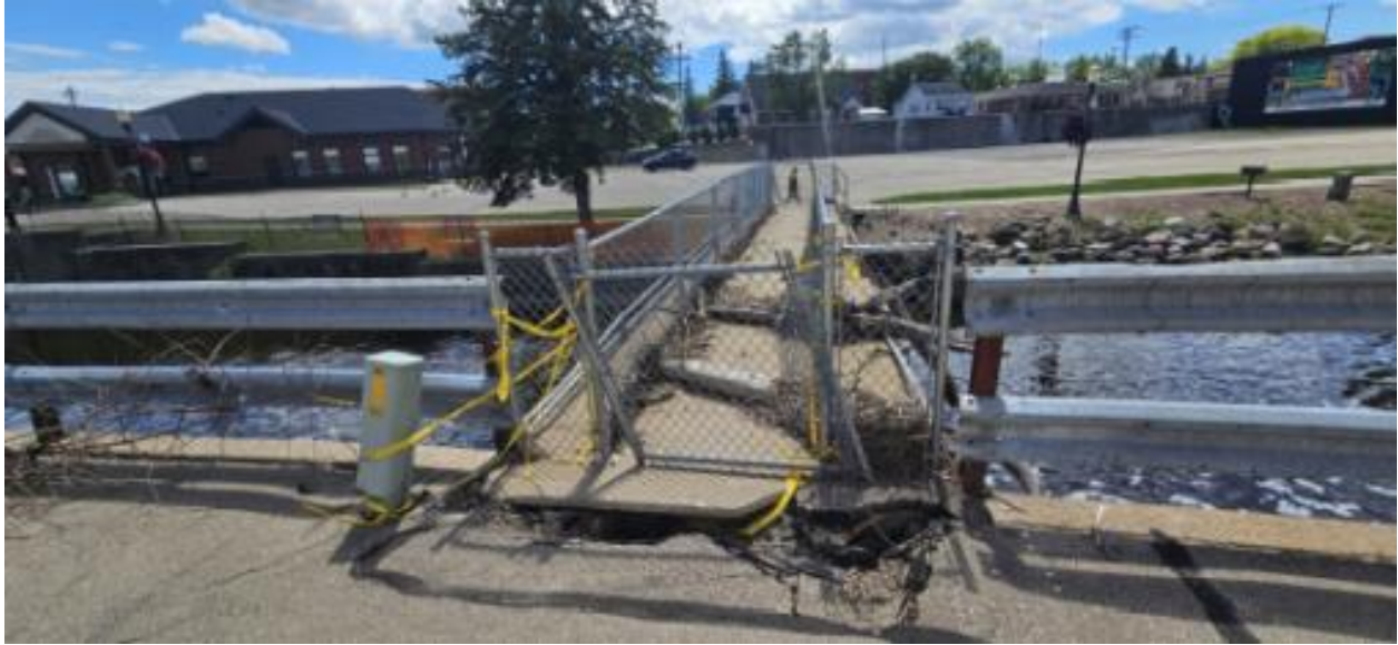
North side of Bridge showing washout over Retaining Wall / Abutment
